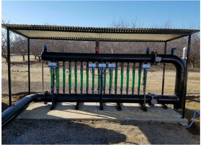
Aqua4D installation at a California almond grower.
